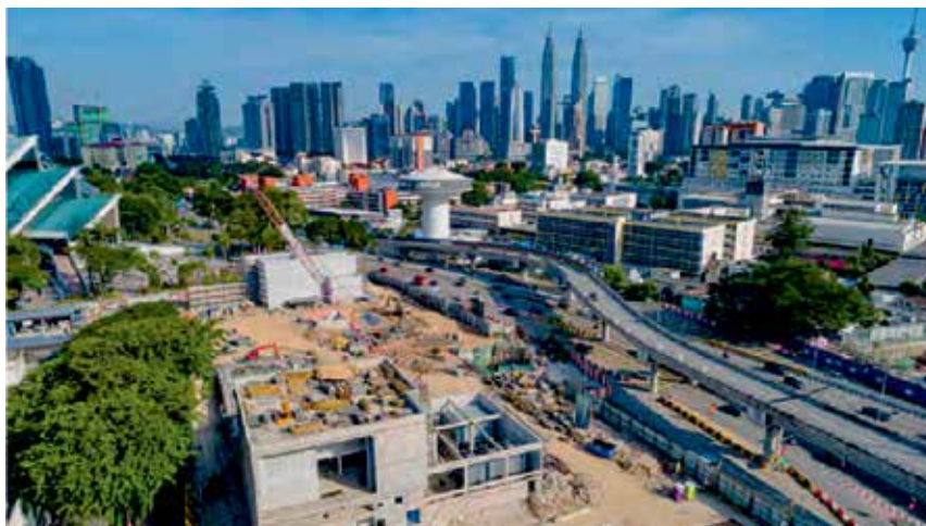
Works progressing smoothly next to a busy highway at the Hospital Kuala Lumpur MRT Station worksite
