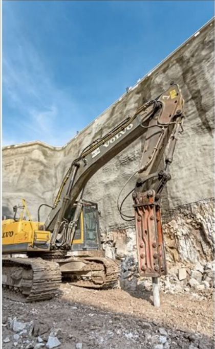
Ground conditions in the KL city centre are a volatile mix of granite, karstic limestone and Kenny Hill formation. If not managed properly in planning and during construction, ground movements or sinkhole occurrences could bring dire consequences to lives and properties.
