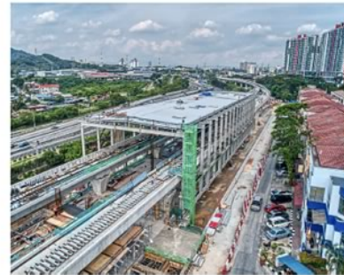
The MRT Damansara Damai station is currently undergoing architectural and system works fit out for station structures, including entrances, link bridges, an access road and walkway.
