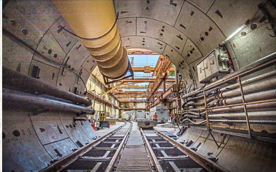
Ten tunnel boring machines are now mining concurrently, with two more to be deployed by the third quarter of this year. Tunnelling work is at a painstaking pace of 7m per day.
