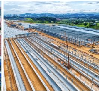
The 67ha Serdang Depot which can house 32 trains will receive its first train in 2020. A section of the depot has already undergone system track works.
